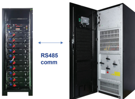
U-EQ33 UPS + lithium batt system
